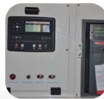
Control Panel & MCB
